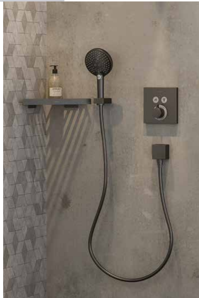
Products shown: Square Select concealed valve with Raindance (300) overhead and Select hand shower (88102090)
